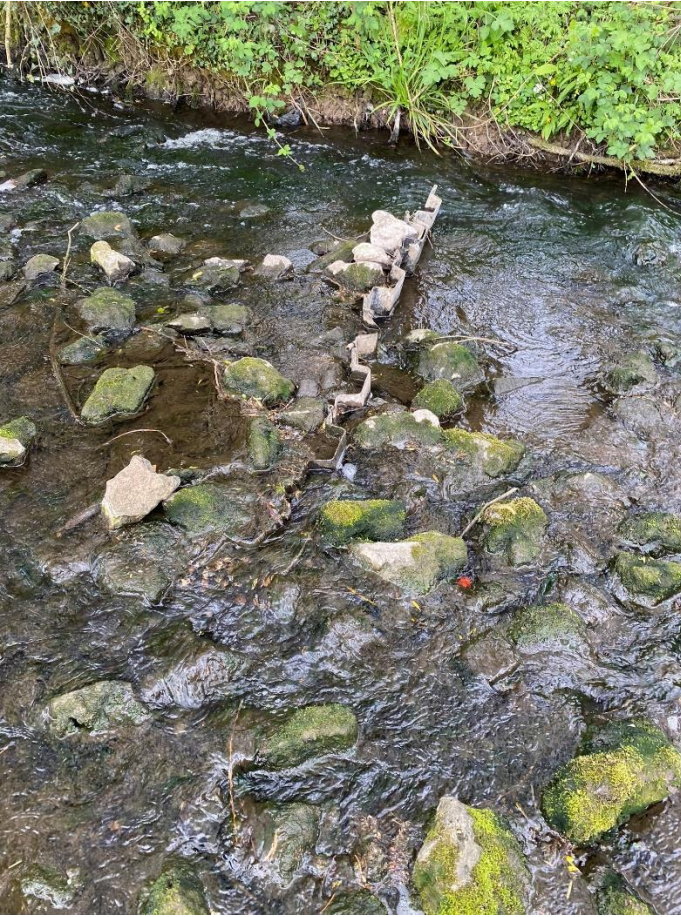
Figure 2.8. General composition of rock ramp feature and exposed sheet piling at downstream end of feature
